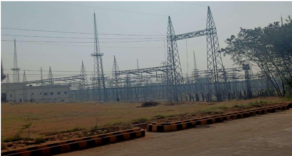
Fig. Power Distribution Plant
